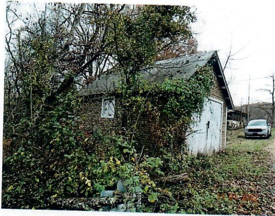
B. 3 dilapidated wooden framed sheds and storage buildings filled with trash and debris.
